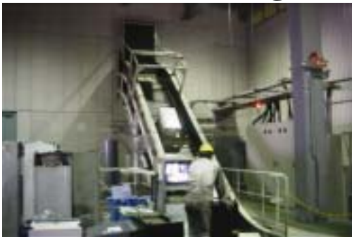
The thermal insulators and Freon recovery facility
